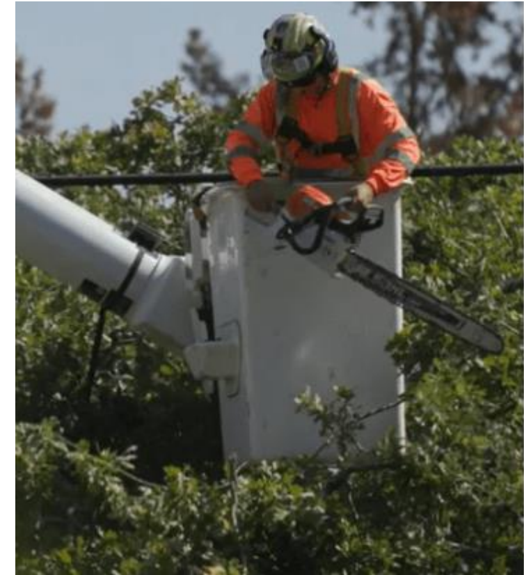
Powerline Tree Work
