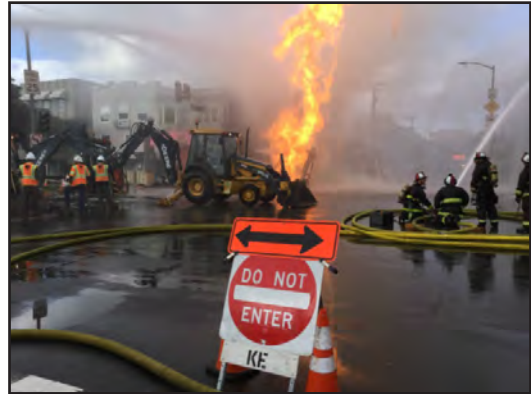
Photo: NTSB report, provided by PG&E
