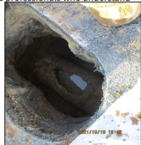
Irrigation pipeline damaged by a D-03 Awnings licensed contractor. From Investigation 21LA01483.
